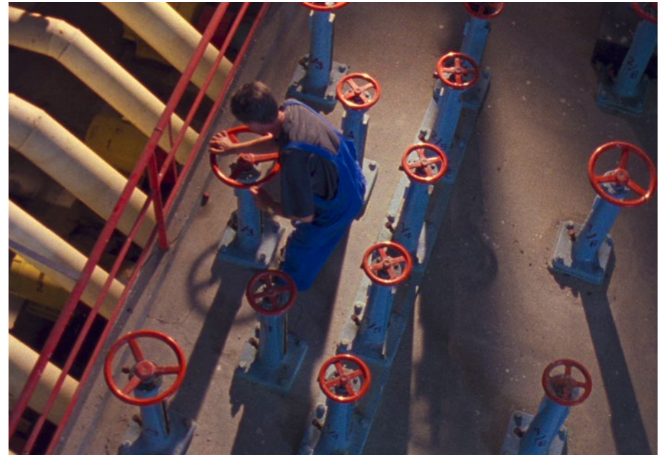
Still from Switch Center
